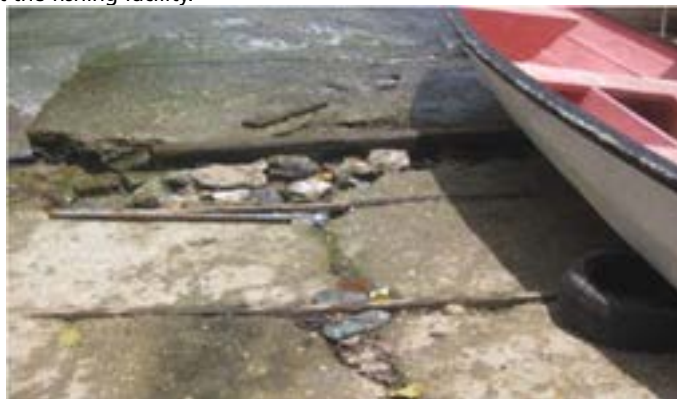
Figure 1: Defective ramp at the Blanchisseuse Fishing Facility.
